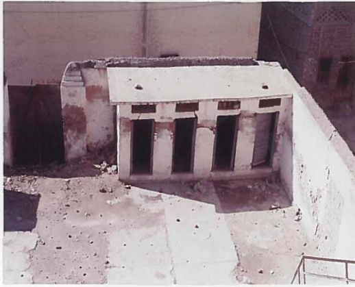
Figure 13. Cracks Abandoned Latrines located at bottom of the mound, Baba Fareed Shrine
