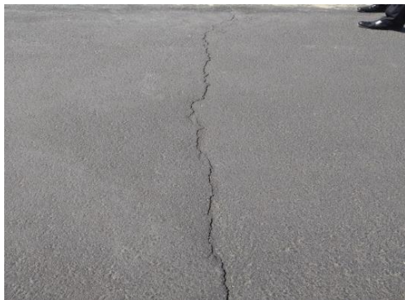
Figure 5. Runway cracks at PAF Base at Bholari
