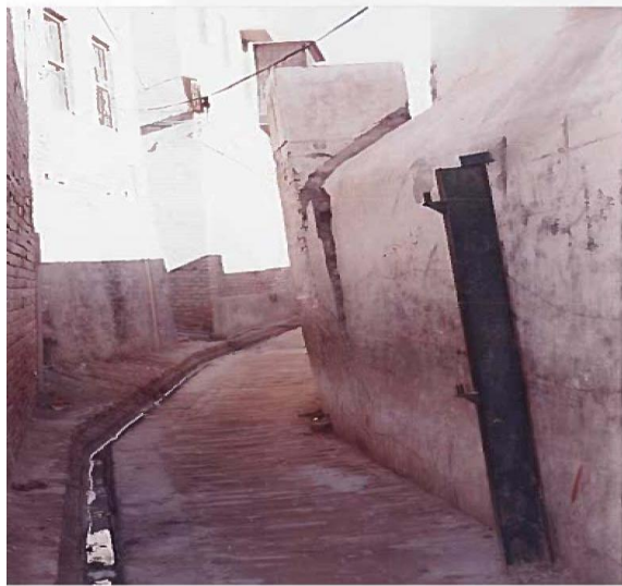
Figure 3. Wall movement of an existing structure at Pakpattan
